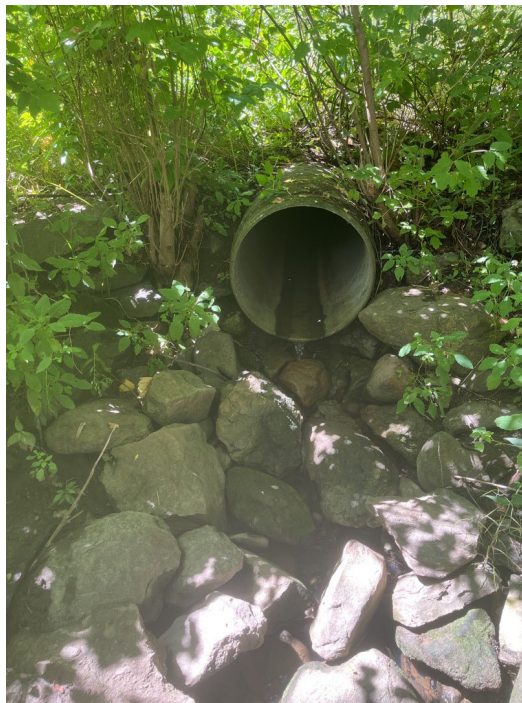
Figure 4. Outfall 40, discharging stormwater runoff from North Elm Street and the Four Winds Apartment, discharging to Stevens Brook.
