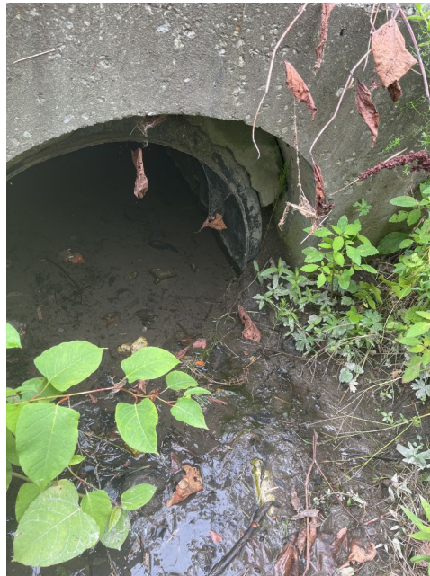
Figure 2. Outfall 38 collecting a portion of stormwater runoff from Aldis Street and discharging to Stevens Brook.
