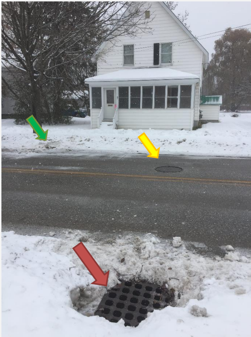
Figure 1: Picture taken facing 67 North Elm Street (white house in the background). The catch basin in the foreground (red arrow) is directly connected to both the storm and sanitary sewers. The lower pipe in the catch basin flows directly to the sanitary manhole (yellow arrow). The catch basin in the background (green arrow) is not connected to the sanitary system.
