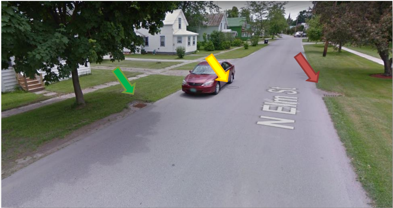
Figure 2: Image from Google StreetView. The red arrow indicates the catch basin connected to both the sanitary and storm sewers. The yellow arrow indicate the sanitary sewer manhole to which the catch basin is connected. The green arrow indicates the catch basin that is not connected to the sanitary sewer.
