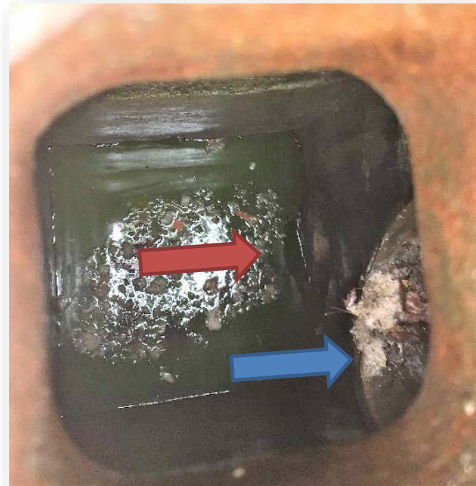
Figure 3: Picture of the catch basin connected to both the sanitary and storm sewers. The red arrow is pointing to the pipe that is directly connected to the sanitary sewer (lower pipe). The blue arrow points to the pipe that leads to the stormwater sewer. In runoff events most runoff would go into the sanitary sewer.
