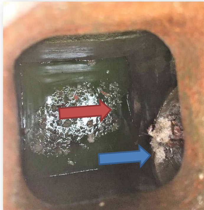
Figure 3: Picture of the catch basin connected to both the sanitary and storm sewers. The red arrow is pointing to the pipe that is directly connected to the sanitary sewer (lower pipe). The blue arrow points to the pipe that leads to the stormwater sewer. In runoff events most runoff would go into the sanitary sewer.
