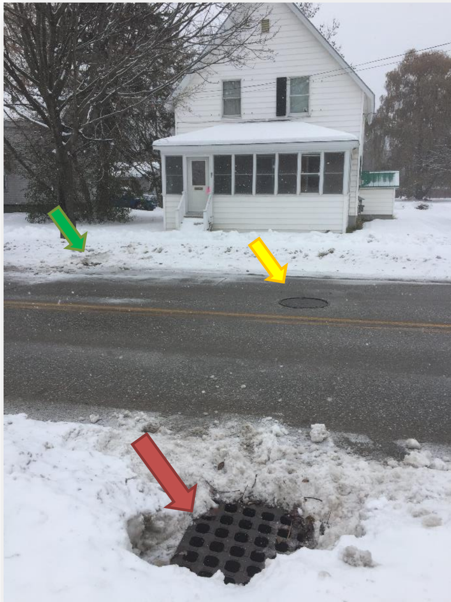
Figure 1: Picture taken facing 67 North Elm Street (white house in the background). The catch basin in the foreground (red arrow) is directly connected to both the storm and sanitary sewers. The lower pipe in the catch basin flows directly to the sanitary manhole (yellow arrow). The catch basin in the background (green arrow) is not connected to the sanitary system.
